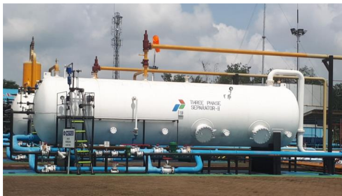
Gambar 1 Separator Tank FWKO
